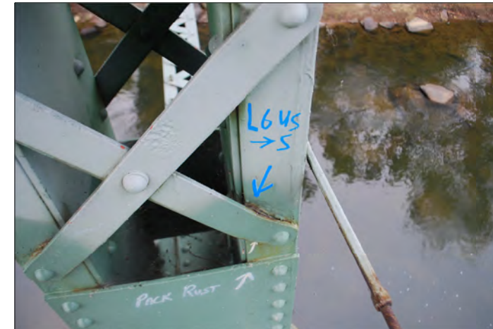
TYPICAL PACK RUST BETWEEN LACING BARS AND TRUSS MEMBERS
