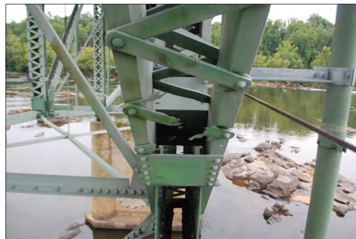
TYPICAL 100% SECTION LOSS OF LACING BARS AND BATTEN PLATES
