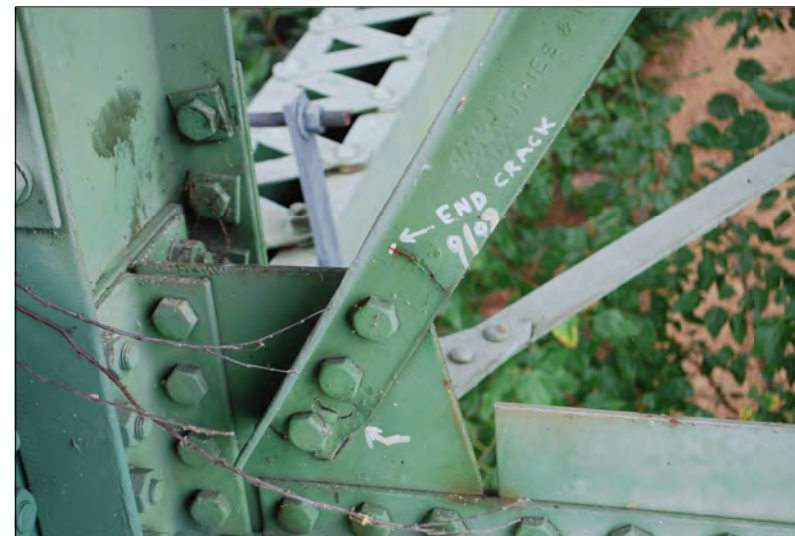
UNIT 13 CRACKED ANGLE
