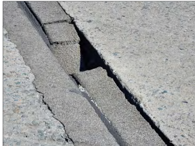
Bridge 11 - North abutment deck joint. Records indicate that the original transflex joint was removed in 2001. At that time, localized repairs were performed using Silspec 900 polymer system where deck header concrete had failed.
