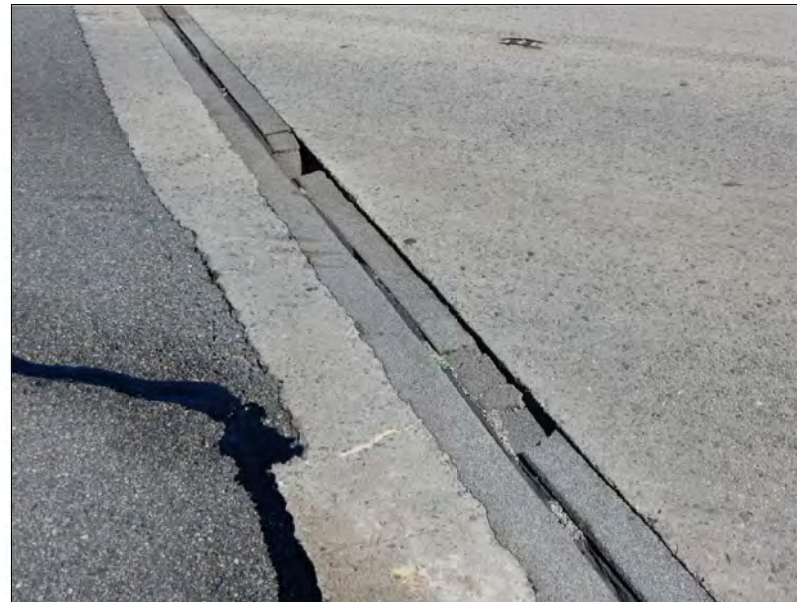
Bridge 11 - The proposed repair to be performed at identified failure locations. The measure length for pricing purposes will be 12 LF. If additional joint failure length is identified and approved by the Engineer, payment shall be made on a per-foot basis, based on the original lump sum bid divided by 12.
