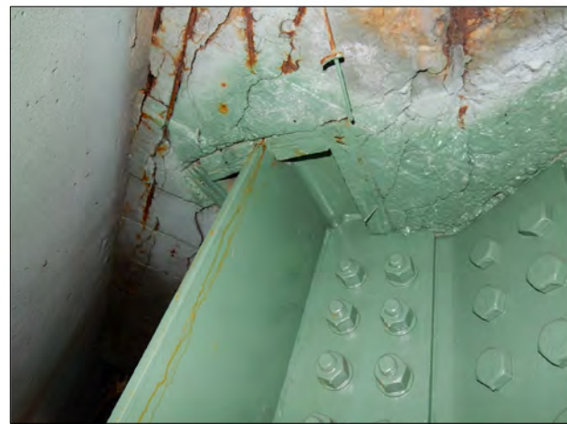
BRIDGE 17 - DECK SOFFIT AT SOUTH ABUTMENT PREVIOUS REPAIR CONCRETE CAST AGAINST BACKWALL
