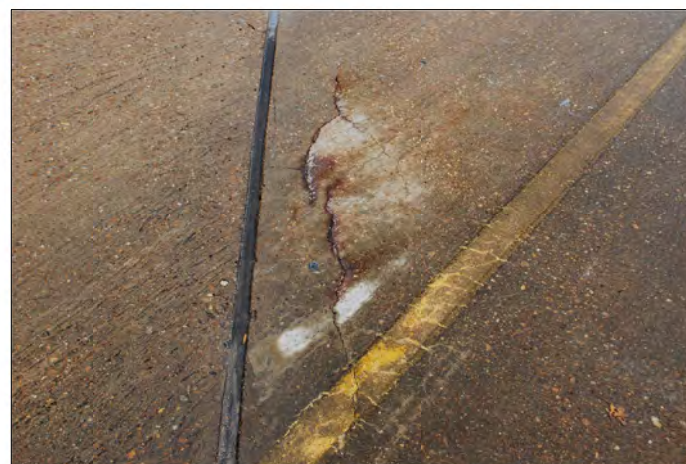
BRIDGE 17 - PIER 2 - DECK SURFACE CRACKING
