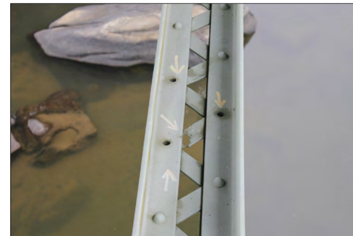
TYPICAL SECTION LOSS OF LACING BARS AND MISSING RIVETS ON TRUSS LOWER CHORD
