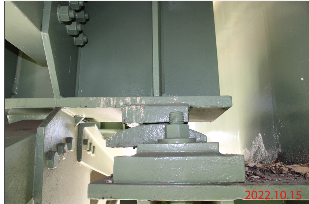
BRIDGE 68 PIER 19, UNIT 2 TYPICAL MISALIGNED BEARING
