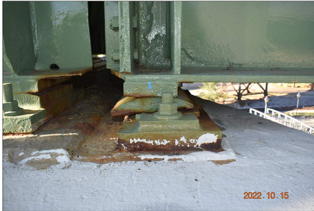
BRIDGE 63, PIER 22, UNIT 22, GIRDER 1 MISALIGNED BEARING
