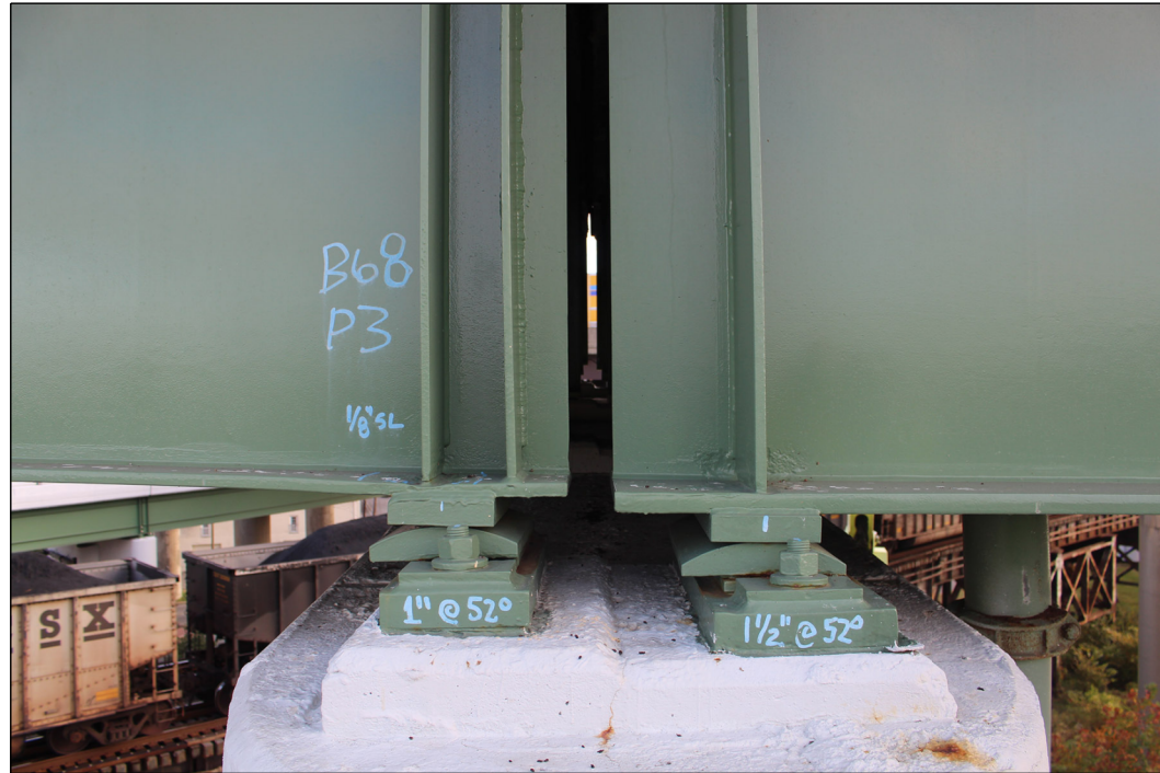
BRIDGE 68 PIER 3, UNIT 6 TYPICAL MISALIGNED BEARINGS
