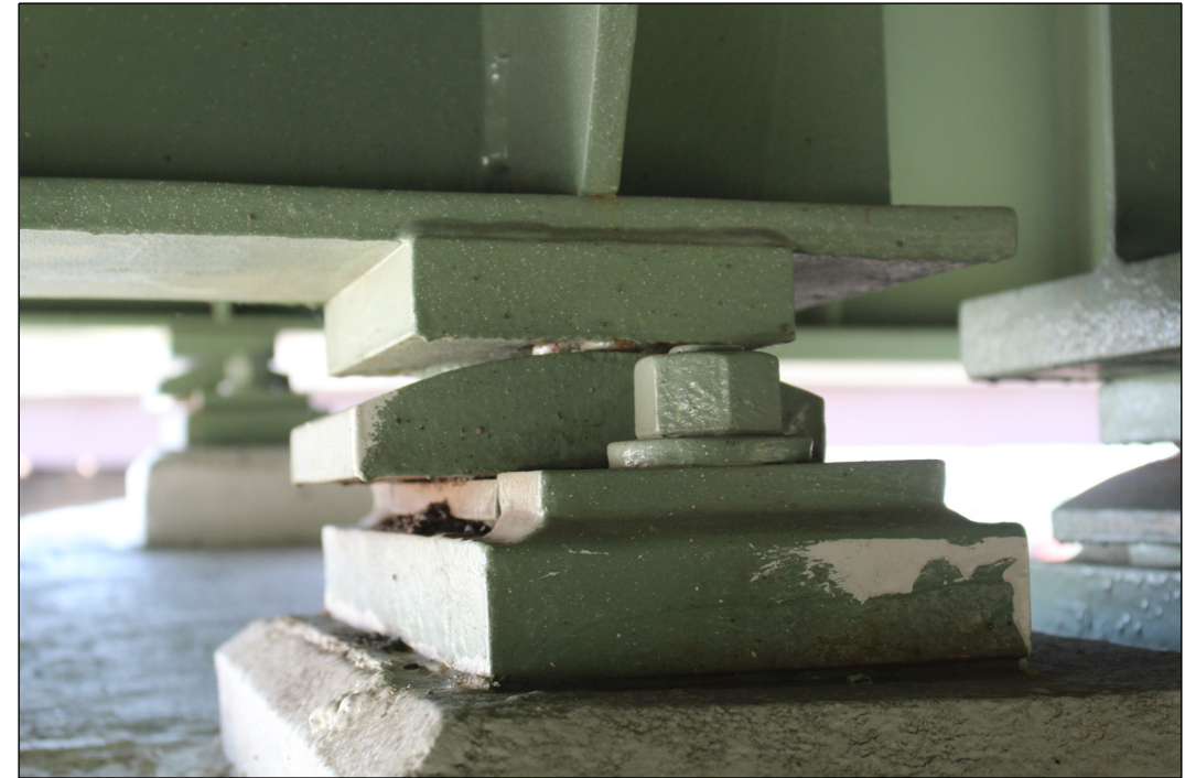
BRIDGE 68 PIER 3, UNIT 6 TYPICAL MISALIGNED BEARING
