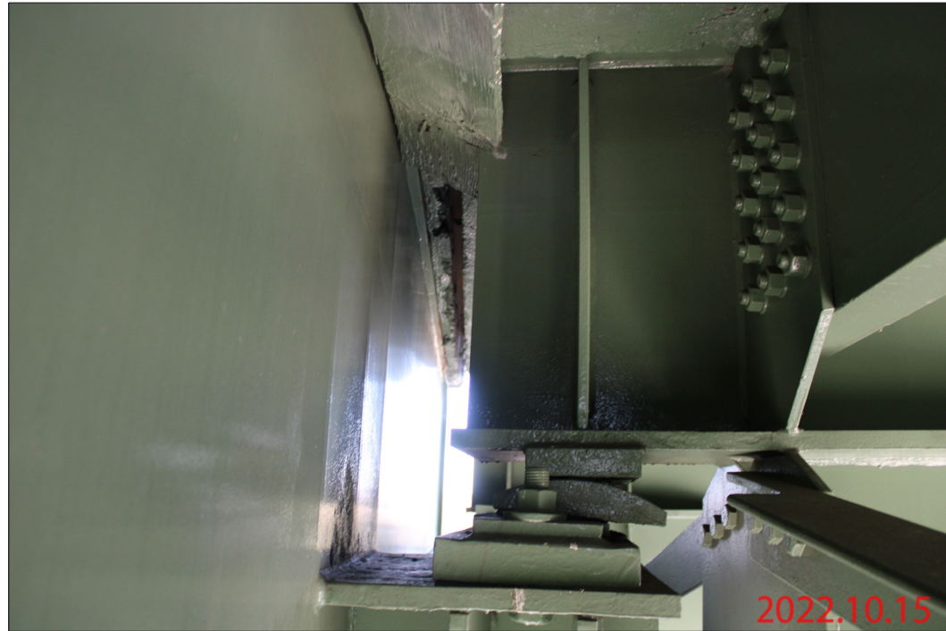
BRIDGE 68 PIER 19, UNIT 2 TYPICAL MISALIGNED BEARING
