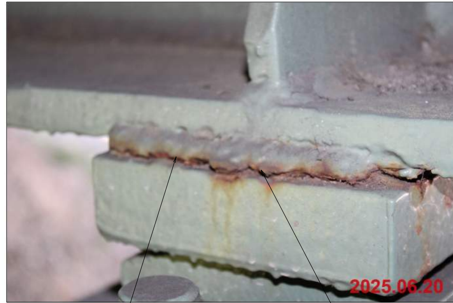
BRIDGE 6 UNIT 4, PIER 3, BEAM 4 TYPICAL CRACKED SOLE PLATE WELD
