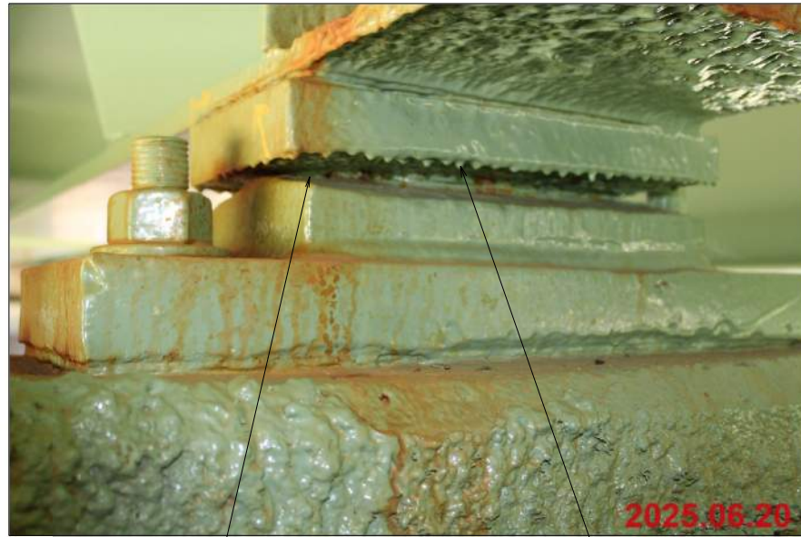
BRIDGE 17 UNIT 4, PIER 3, GIRDER 7 TYPICAL CRACKED SOLE PLATE WELD
