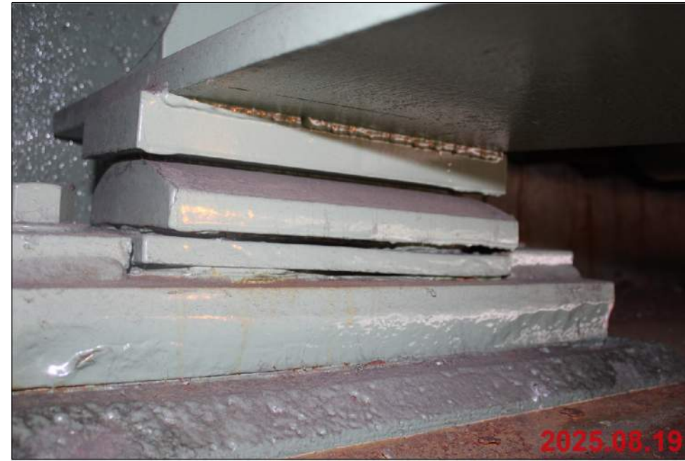
BRIDGE 60 NORTH ABUTMENT TYPICAL MISALIGNED BEARING
