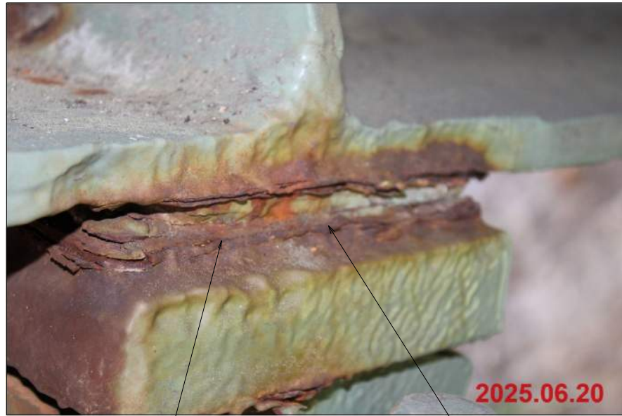
BRIDGE 6 UNIT 4, PIER 3, BEAM 6 TYPICAL CRACKED SOLE PLATE WELD (UNIT 4, PIER 3, BEAM 5 SIMILAR)
