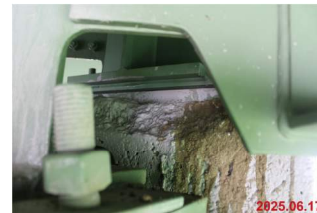
TYPICAL BEARING PEDESTAL SPALL
