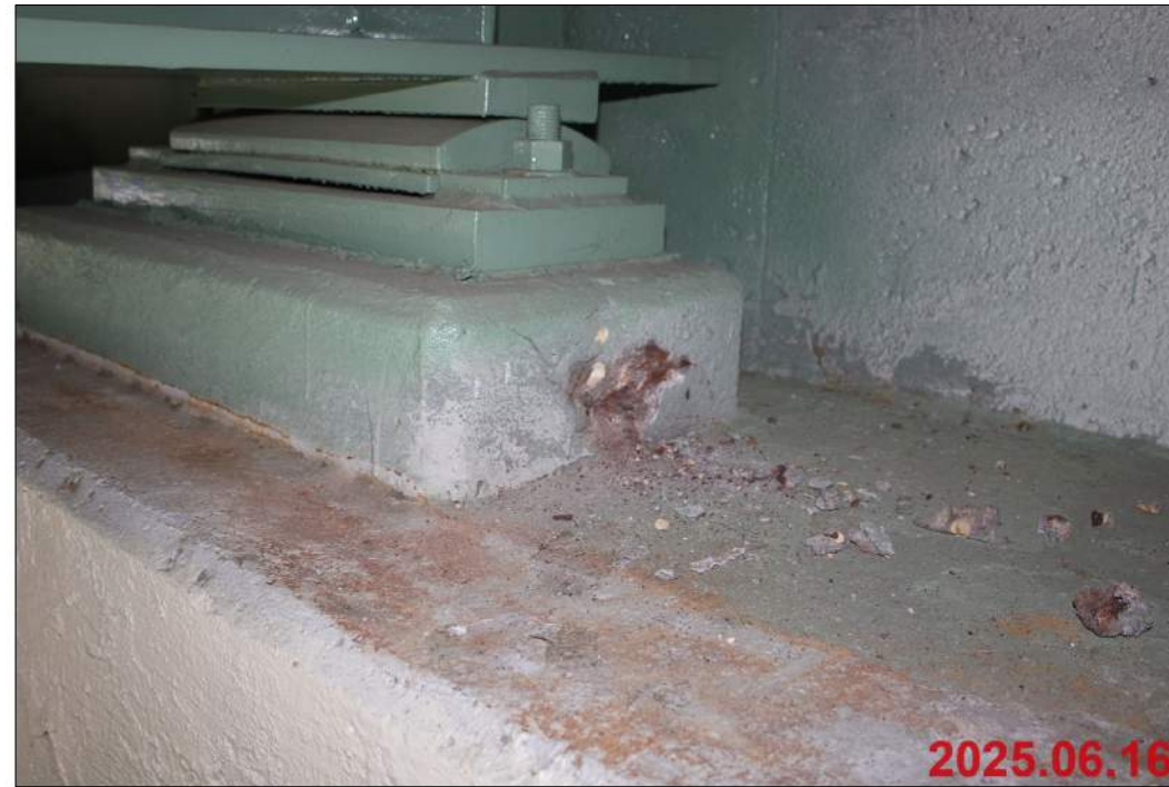
BRIDGE 56 SOUTH ABUTMENT TYPICAL MISALIGNED BEARING
