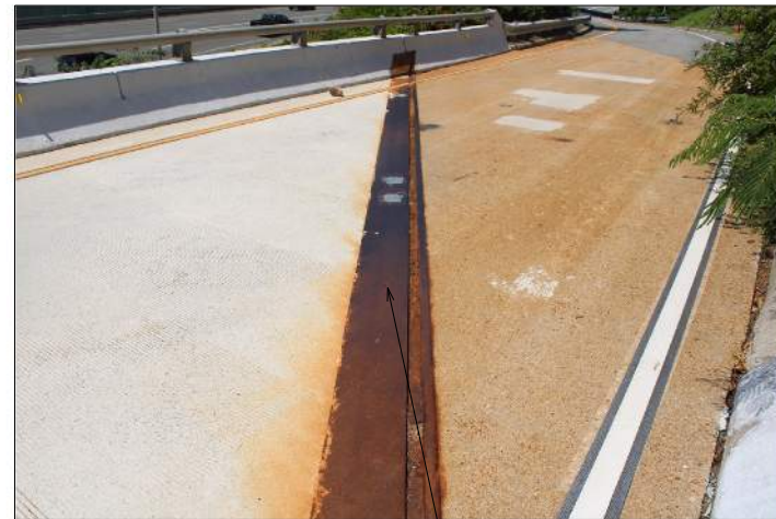
100% LOCALIZED SECTION LOSS IN SLIDING PLATE JOINT
