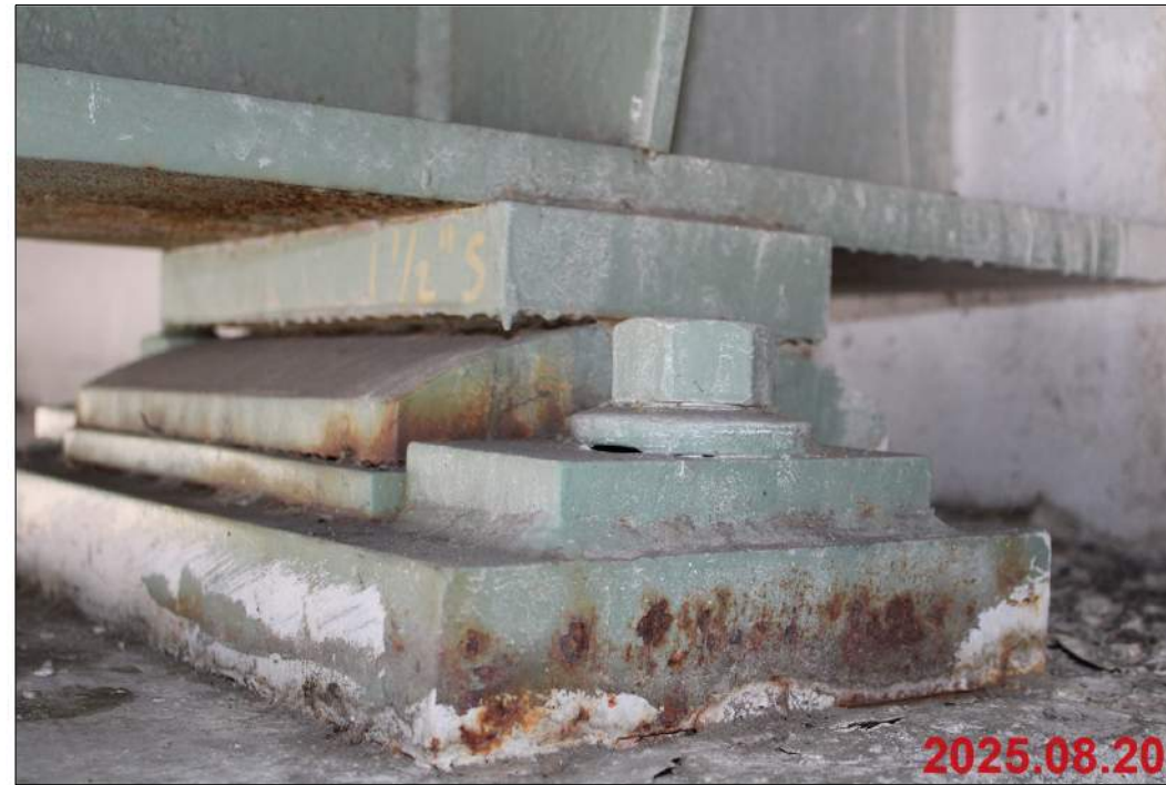
BRIDGE 49 SOUTH ABUTMENT TYPICAL MISALIGNED BEARING
