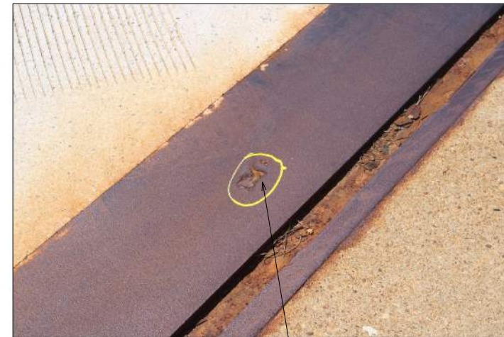
100% LOCALIZED SECTION LOSS IN SLIDING PLATE JOINT
