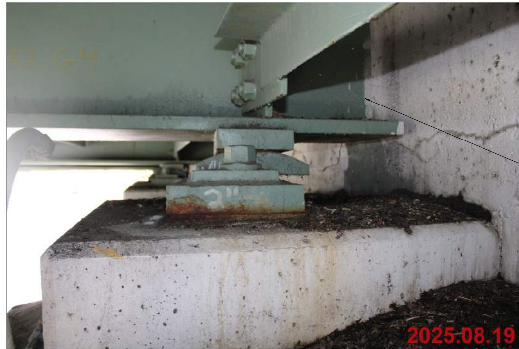
BRIDGE 48 NORTH ABUTMENT TYPICAL MISALIGNED BEARING
