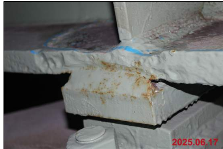
BRIDGE 4, UNIT 1, PIER 1, GIRDER 1 PACK RUST BETWEEN SOLE PLATE AND BOTTOM FLANGE OF GIRDER
