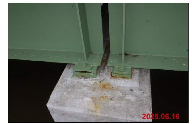
TYPICAL BEARING PEDESTAL SPALL
